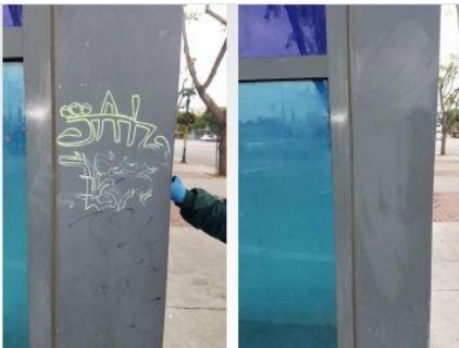
Cleaning up vandalism.
